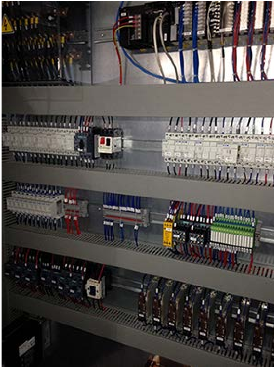
Figure 11: Internal view of the electric control cabinet
