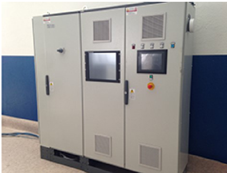
Figure 4: Electrical control cabinet
